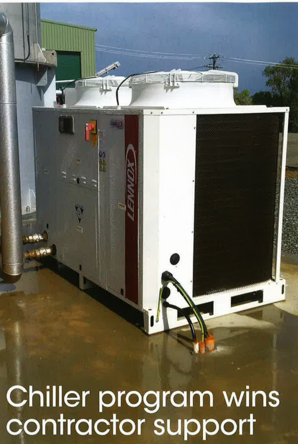
A Lennox Ecolean chiller was installed at the Sanitarium plant in Cooranbong, NSW.
